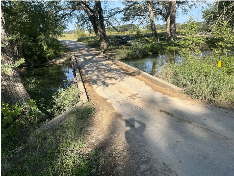
PHOTO 1 Recommended Maintenance Needs
