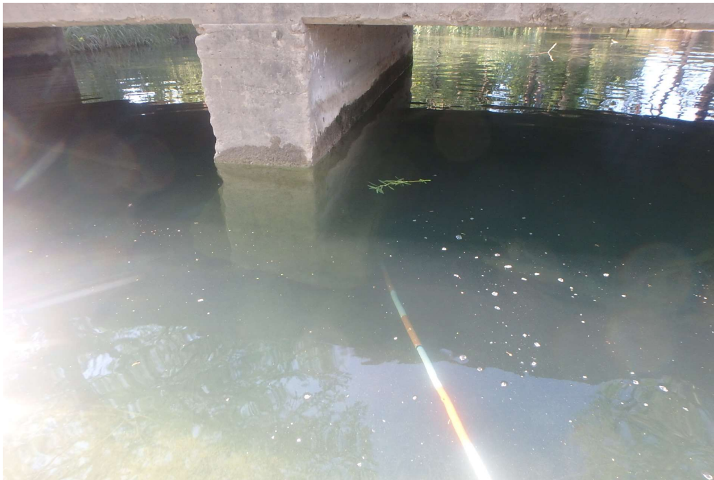
PHOTO 6 Recommended Maintenance Needs
